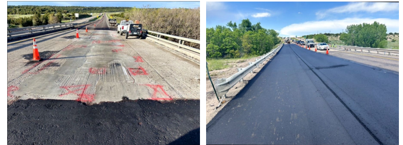
I-25 near Colorado City, Before and After Condition
